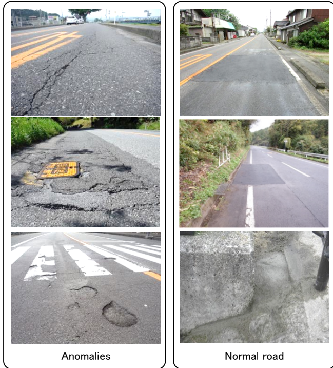
Fig. 4. Examples of reference images collected by the local government of Tottori prefecture for the dataset.
